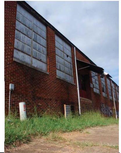
Figure 1.4 - Reusing the community’s empty industrial buildings continues to be a challenge, in Hickory and throughout the Greater Hickory region. 1.1 lists and describes those documents used in the development of this plan.
