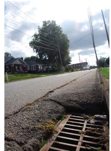
Figure 7.4 – Managing stormwater is a challenge, particularly ensuring that urban runoff is treated adequately before it is discharged into the Catawba River or other local streams.
